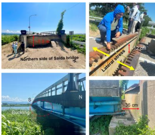
Fig. 3 Damages in the Saida bridge, Uchinada
