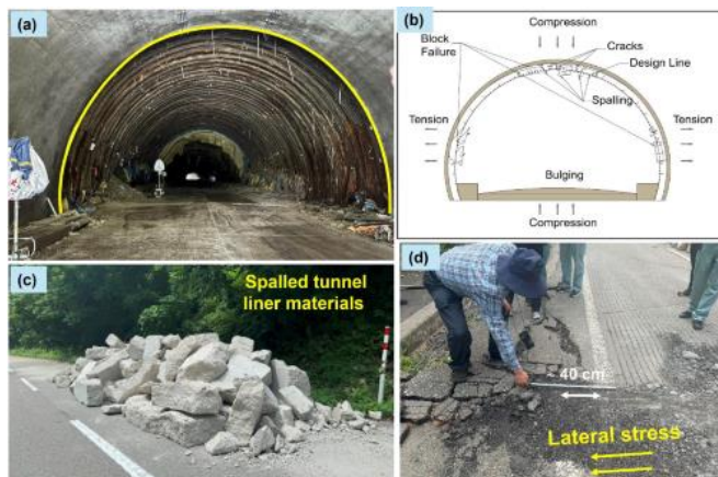
Fig. 6 (a) Tunnel damaged by the sliding mass; (b) schematic diagram of liner spalling; (c) concrete liner mocked out from the tunnel; and (d) lateral slip observed along the roadside near the tunnel entrance (photographs coordinate location: 37° 28' 40.6416" N and 137° 11' 58.7292" E)
