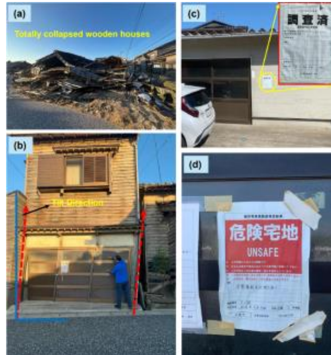
Fig. 7 (a) Completely collapsed building; (b) tilted building; (c) building inspection certificate; and (d) inspection certificate attached to a building suffered with uplift and subsidence.
