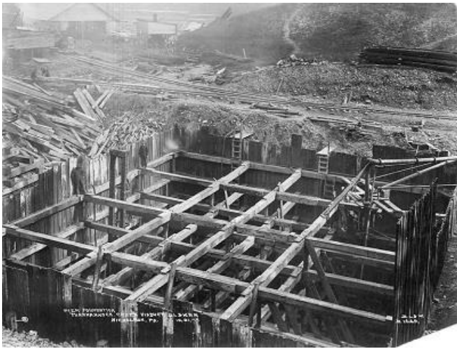
IMAGE 13: Excavation progresses on Pier 5 of the Tunkhannock Viaduct, October 1913. Source: Archives West (2017).
