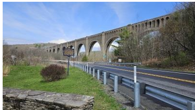
IMAGE 4: The Tunkhannock Viaduct soars over the valley of its namesake creek in Nicholson, PA. Source: Author.
