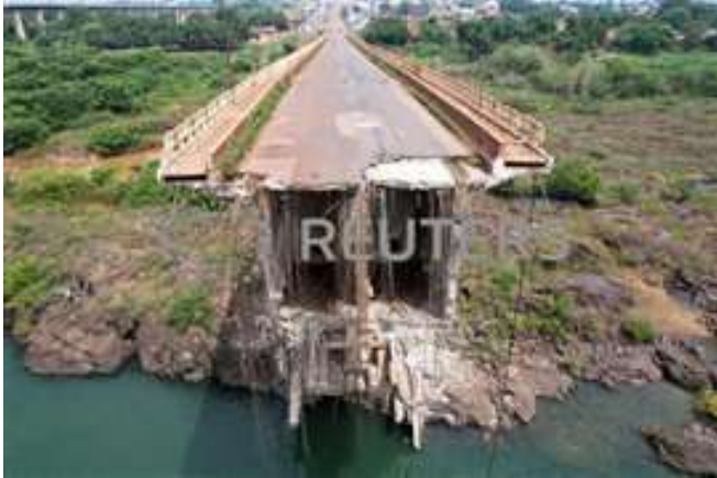
The collapsed Juscelino Kubitschek Bridge in Brazil (Image: REUTERS/Mauricio Marinho)
